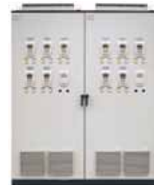
LV Distribution Panels
